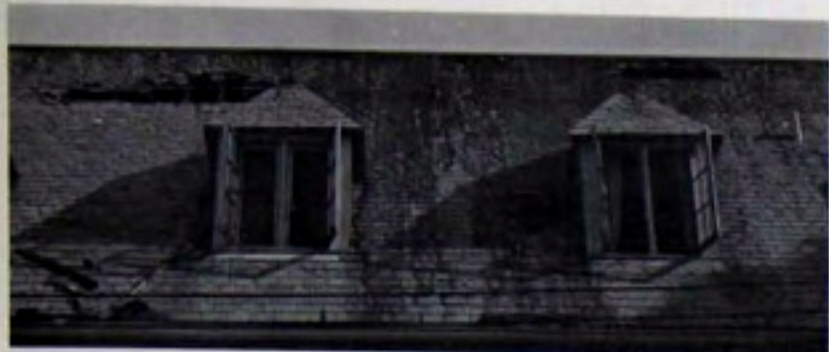
FIRE DAMAGE as seen from the outside of the House
